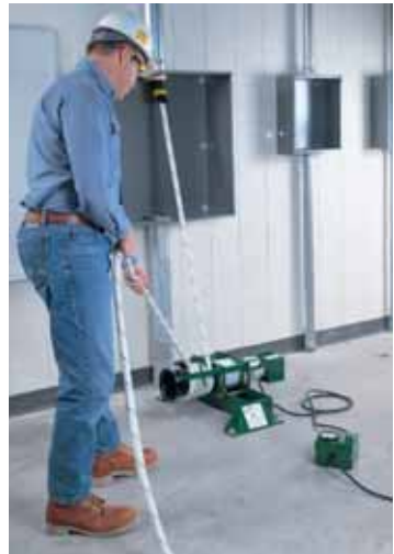
Ultra Tugger™: Use via floor device.
